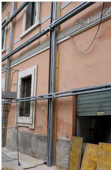
Figure 30: L'Aquila, Italy October 2011. Cold-formed steel channel waling and soldiers with threaded rod transverse ties. Note: this type of temporary work can encroach onto footpaths and road corridors, which can be an issue if there is limited space. (Photo: Win Clark)
