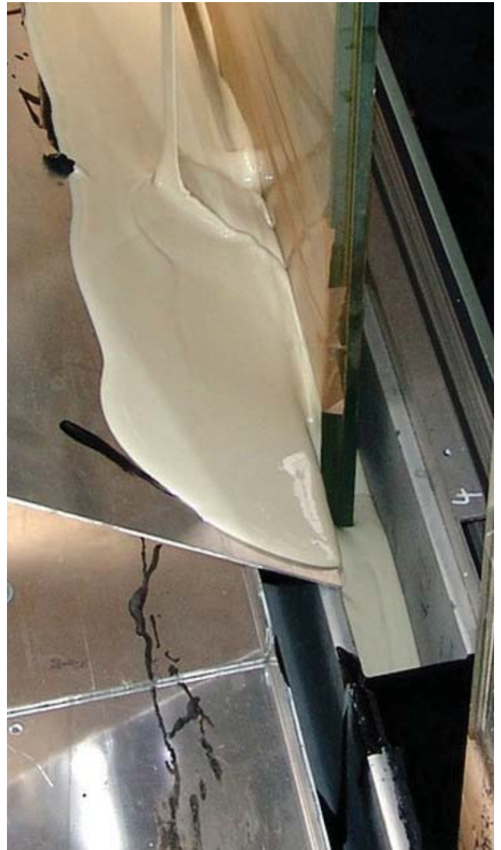
Picture 8: Easy injection of SikaGlaze GG-735 by using a sloped metal sheet
