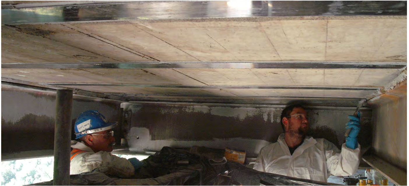
Sika Approved Contractors BBR Contech install Sika CarboDur plates to strengthen the Mohaka River Bridge.
