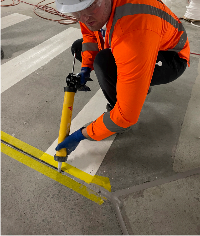
Progress shot: Sikaflex® PRO-3 Purform® being installed for its high movement capability and good durability
