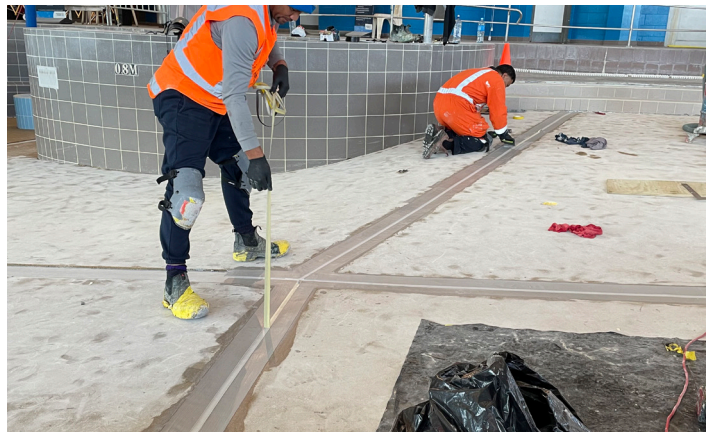
During: Installation of Sikadur® Combiflex SG, a high performance joint sealing system was used to replace the deteriorated joints.
