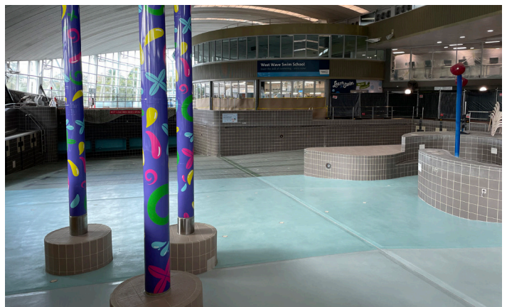
Completion: All joints on the base of the pool were replaced with Sikadur® Combiflex SG, a long term solution used in swimming pools.
