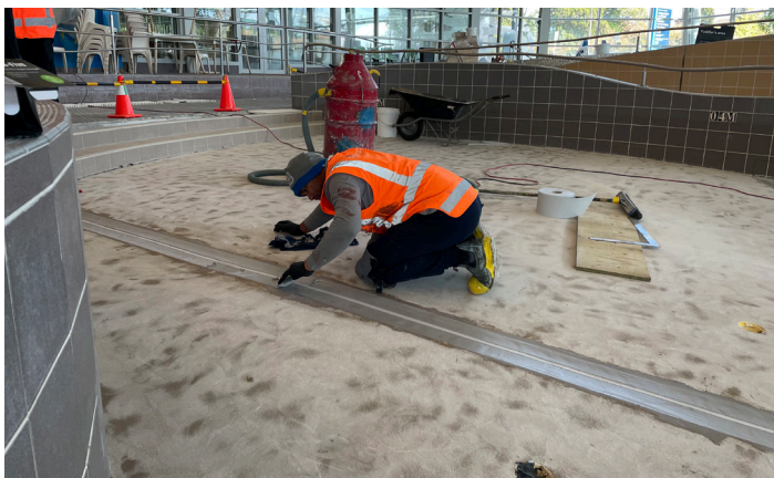
During: Topcoat securing Sikadur® Combiflex SG in place with Sikadur®-31 a structural epoxy adhesive.
