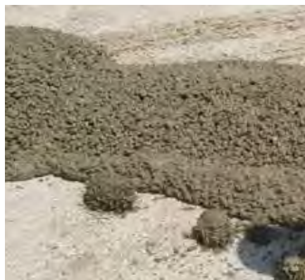
Figure 4.1.2: Fresh concrete with balling
