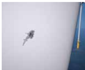
Structural composite damage.
