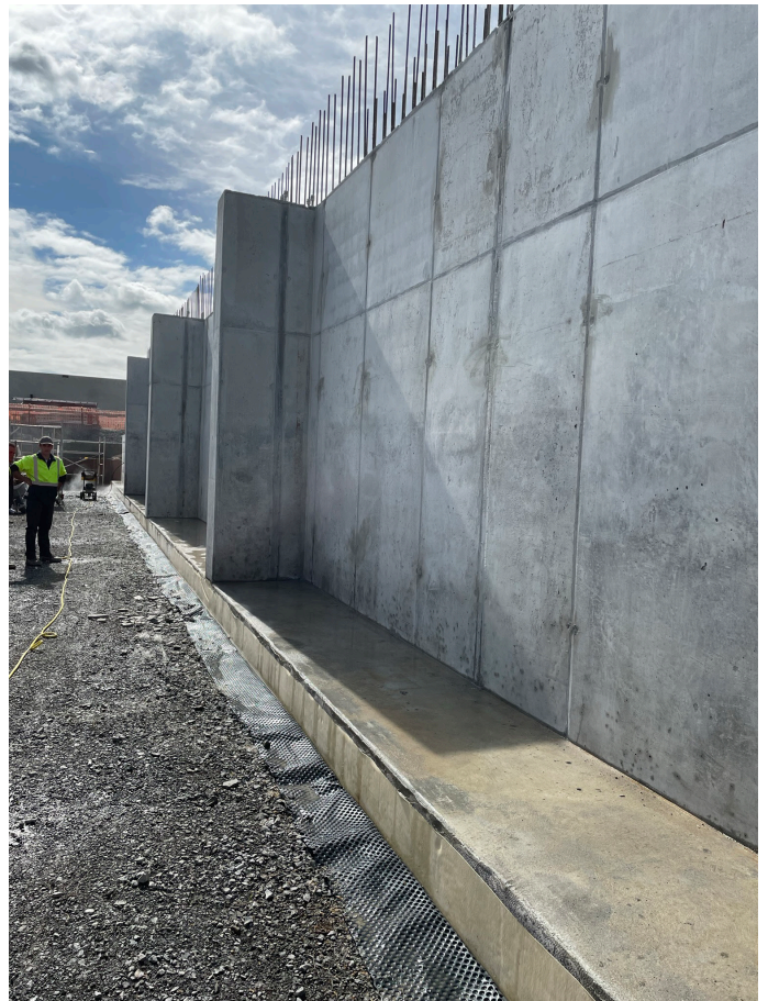
In situ concrete walls prior to SikaProof® P-12 installation. SikaProof® A+ 12 visible to edge of footing.
