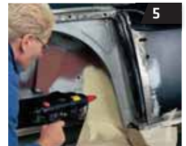
Reproducing the original factory underseal following repairs to door sills front and rear valances.
