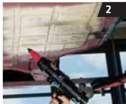
Wide angle spray application following repairs to floor pan, luggage compartment floor and wheel arches.
