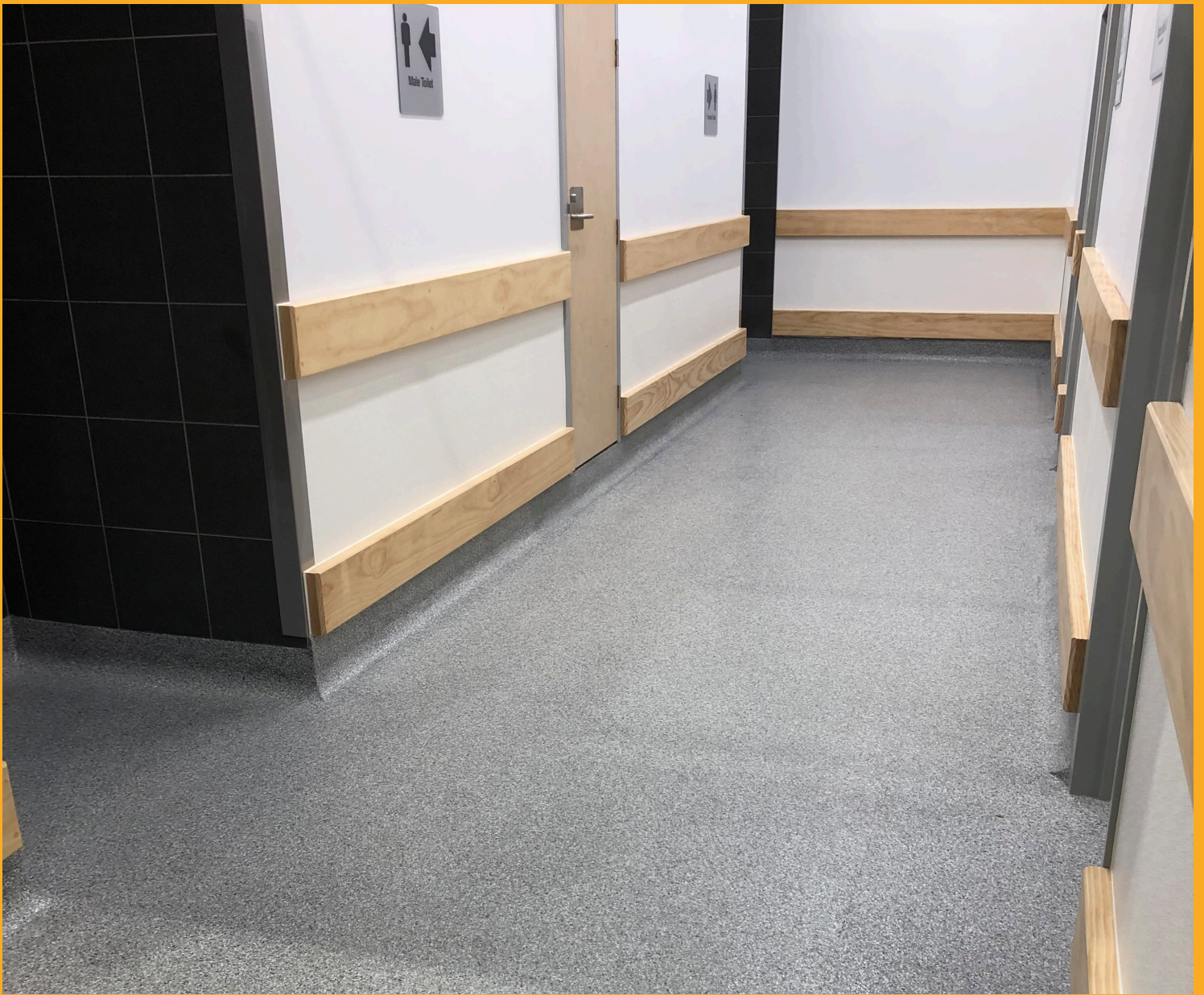
Sikafloor®-264 (Vinyl Chip Flake 'Richmond Marble') - Hallway
