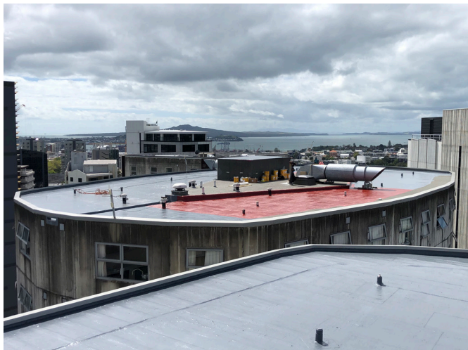
Adjacent Empire building's turn for to get a system coating of SikaRoof MTC (now i-Cure).
