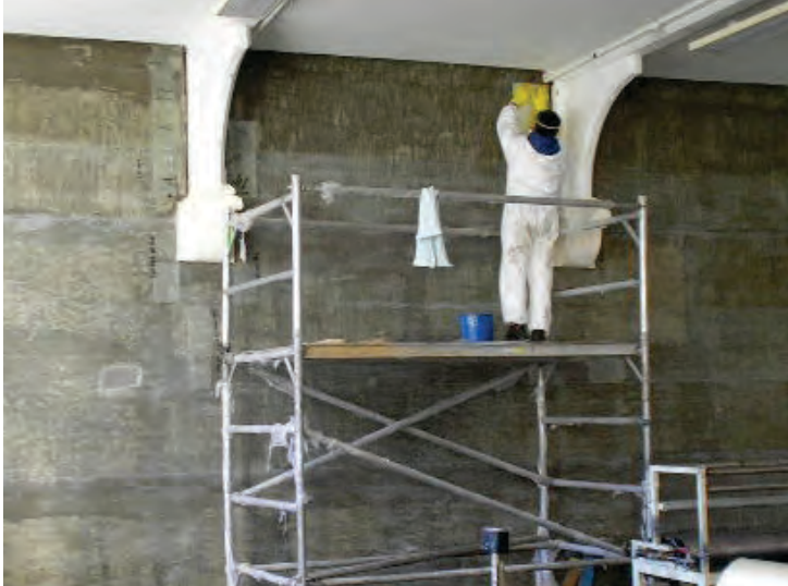
BBR Contech applied SikaWrap-100G fabric seismic strengthening to the historic Arts Centre buildings in Christchurch prior to the devastating earthquakes of 2010 and 2011.
