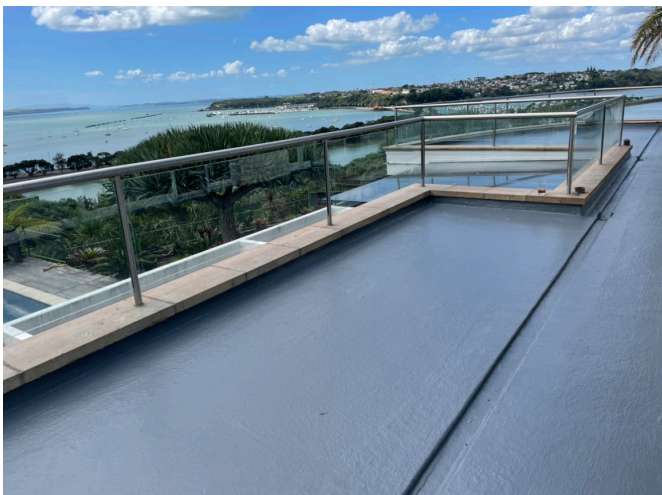
SikaRoof® i-Cure-22 system applied over SikaScreed®-1 on concrete balcony deck over habitable space below.
