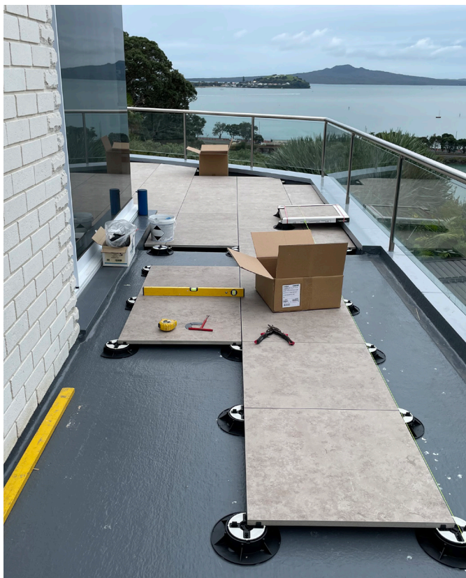
Tiling on pedestals being installed over the SikaRoof® i-Cure-22 system. East side of house.
