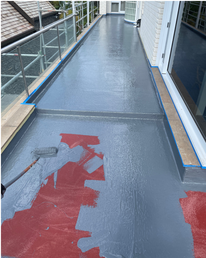
SikaRoof® i-Cure's top coat (Sikalastic®-641) been applied over the system base coat (Sikalastic®-631). East side of house.
