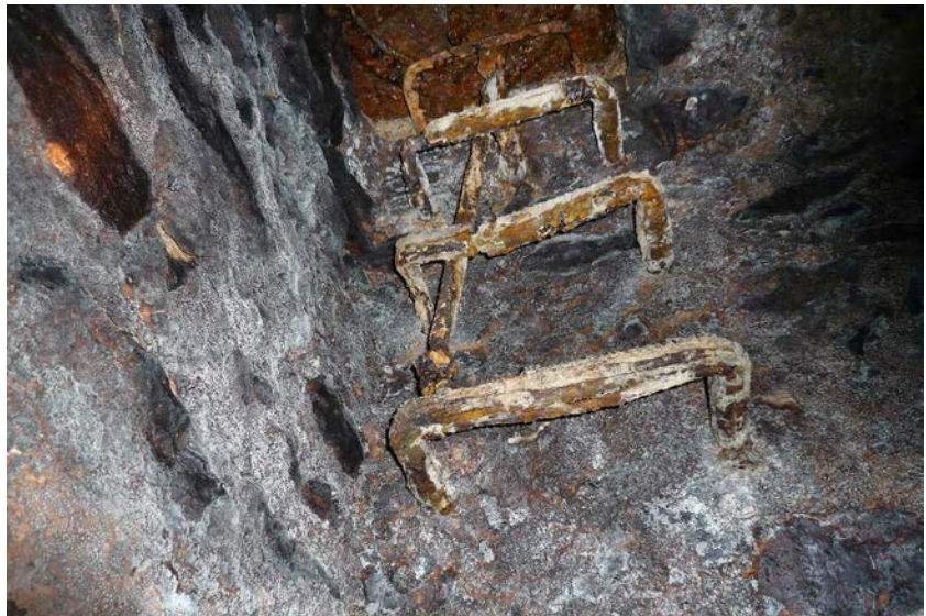
Biogenic sulfuric acid attack
