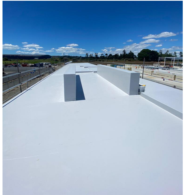
New plant room roof - Sarnafil G 410-20 L Felt. (On right of image, new cool room at floor level not build yet)
