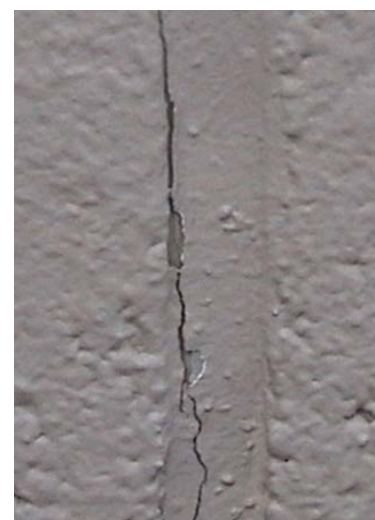
Cracked paint film over joint sealant
