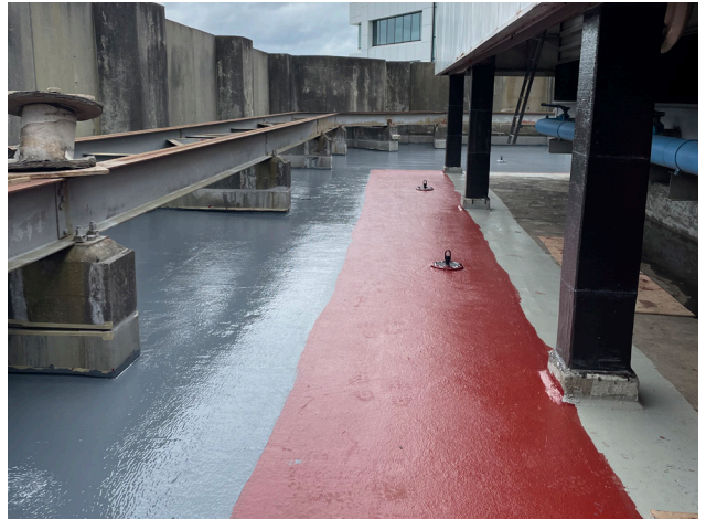
SikaRoof i-Cure Basecoat (Red) has a layer of fibreglas reinforcing imbedded within it. The Topcoat (partially applied) is Slate Grey.
