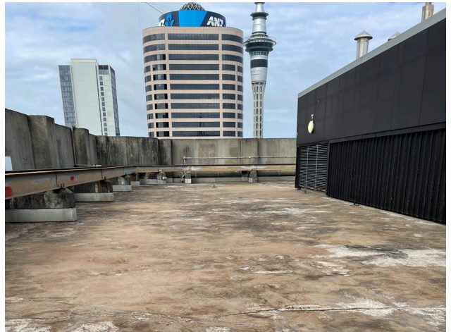
During the preparation of the surface, the original asphalt had to be removed and cracks repaired.
