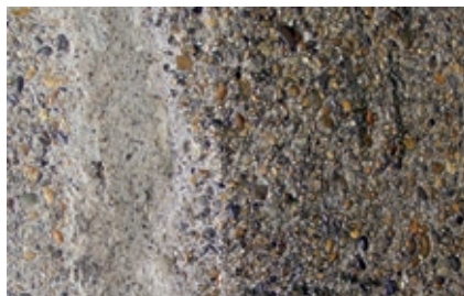
Fig. 8.7.4: Due to continuous exposure, the cement film is eroded in an initial step, and thereafter larger and larger aggregates are rubbed, knocked or washed out of the hardened cement paste.
