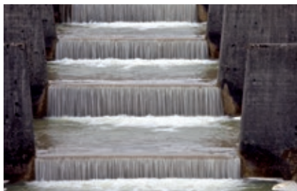
Fig. 8.7.1: Particularly in whitewater, concrete surfaces are subject to massive additional strains by rubble, sharp edges and abrasion, as well as possible temperature stresses due to frost exposure.
