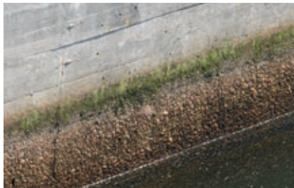
Fig. 8.8.1: Heavy leaching and damage to the structural concrete are observed particularly in the water splash zone of biological treatment basins.
