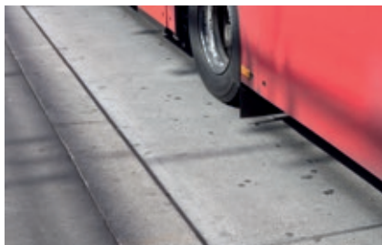
Fig. 8.7.2: Concrete roadways and other publicly accessible areas, especially those experiencing high volumes of traffic or concentrated loads, are subject alongside high mechanical burdens also to strong abrasion, often presenting the risk of a smooth, slick surface.
