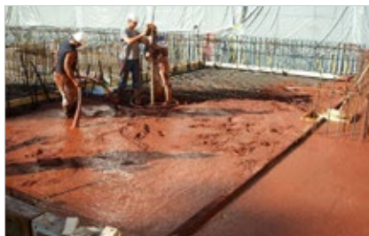
Fig. 8.16.1: The floor, walls and ceiling of this medical building were constructed with heavyweight concrete using hematite metallic aggregates to ensure full and secure radiation protection.
