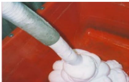
Fig. 8.15.2: Foam generated by a foam generator and SikaPoro® to produce cellular/foam concrete.
