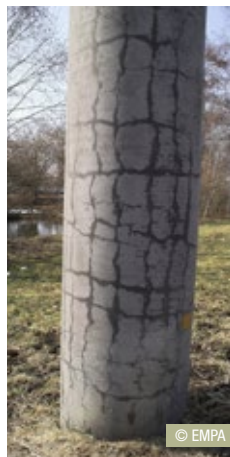
Fig. 8.6.3: The appearance of ASR damage can be assessed very well on the drying concrete surface of this bridge pylon. Damage can appear within years or only after decades.
