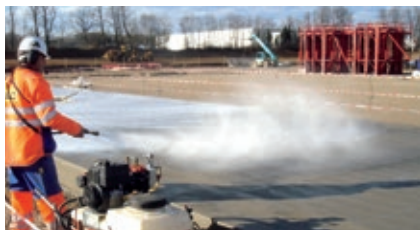
Fig. 8.10.2: Immediate coverage or curing of concrete surfaces exposed to the elements is the most crucial step for protection of such surfaces.
