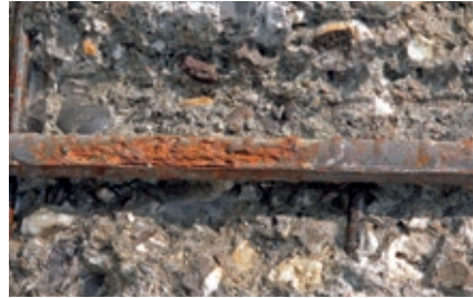
Fig. 8.2.1: Damage to concrete structure due to insufficient concrete cover and low concrete quality.
