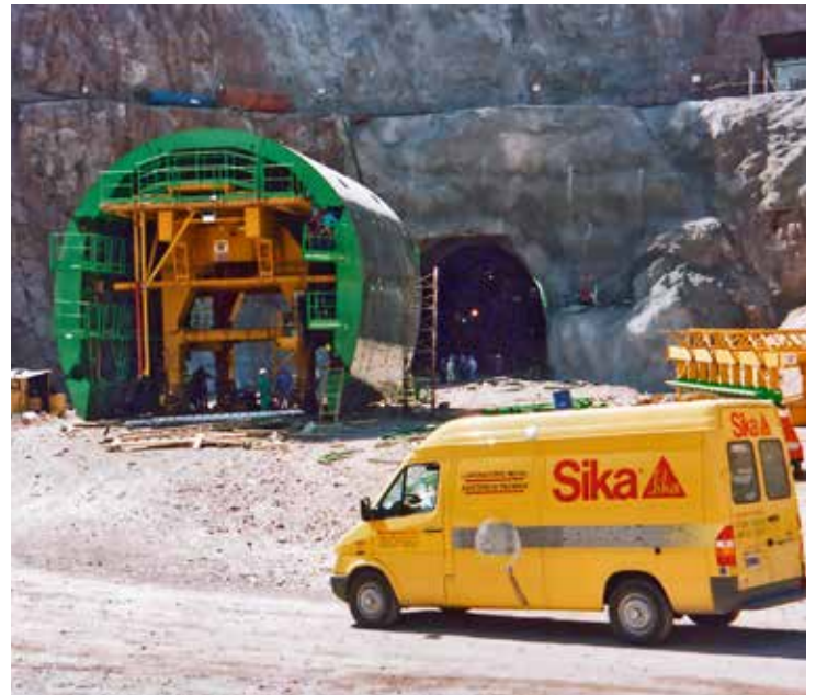
POTRERILLOS HYDROELECTRIC CENTRAL, ARGENTINA
